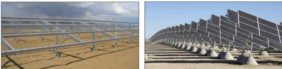
Figure 3. Typical Ground Mounting Solar Panels Structures
